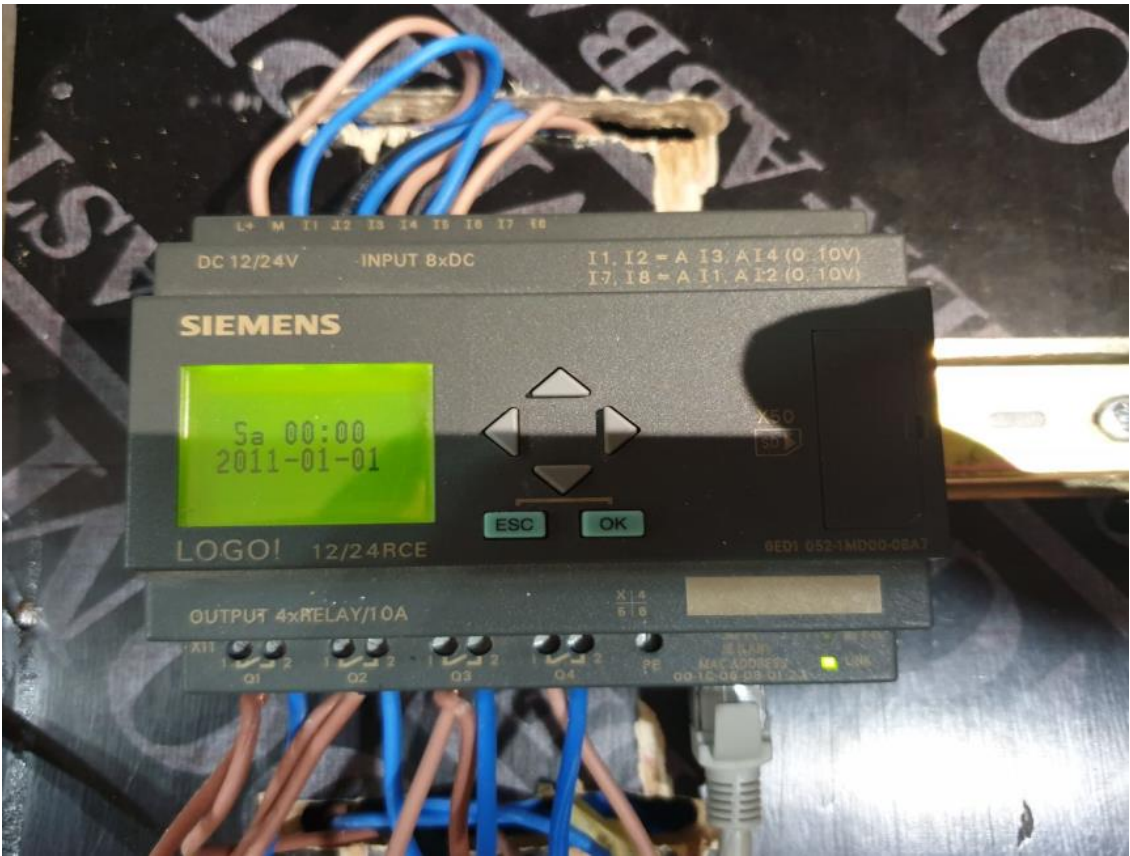
Fig.1 View of PLC used
